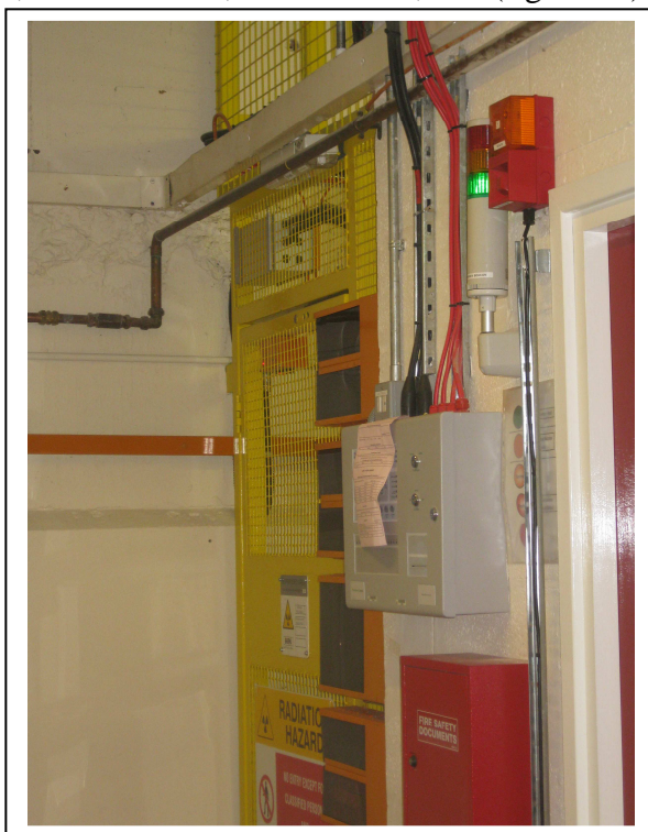
Figure 4.6.1: ODH and LH 2 Beacons outside the Outer Door
