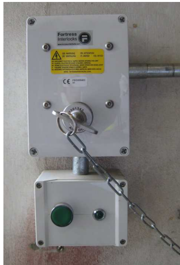
Figure 4.2.6: PPS Solenoid Keyswitch in No Entry state
