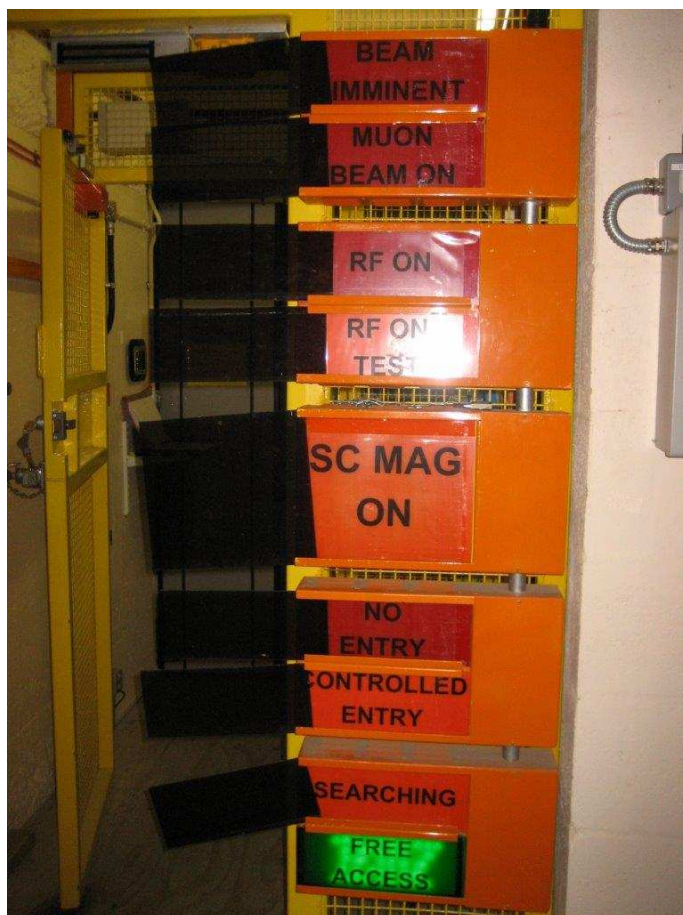
Figure 1.4: PPS Indicator Signs at Controlled Entry Doors. The bottom four indicate the access state.
