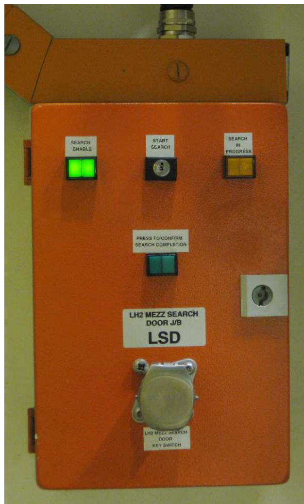
Figure 4.3.2: Search Control Panel (SCP) for LH2 Mezzanine
