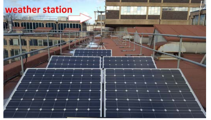
Fig. 2. The studied PV array installed at Brunel University London
