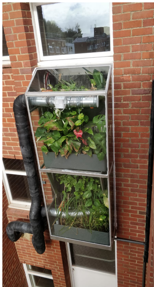
Figure 1: View from the exterior of the Casetta type NBS air filtering unit at Clifton Hall, Brunel University, London
