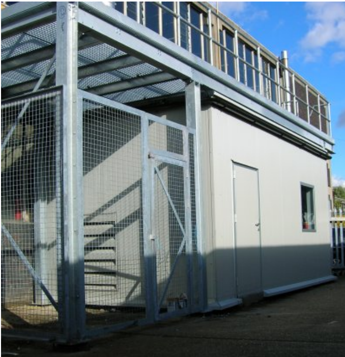
Fig. 5. Newly installed (October 2005) Combined Heat & Power and PV experimental facility.
