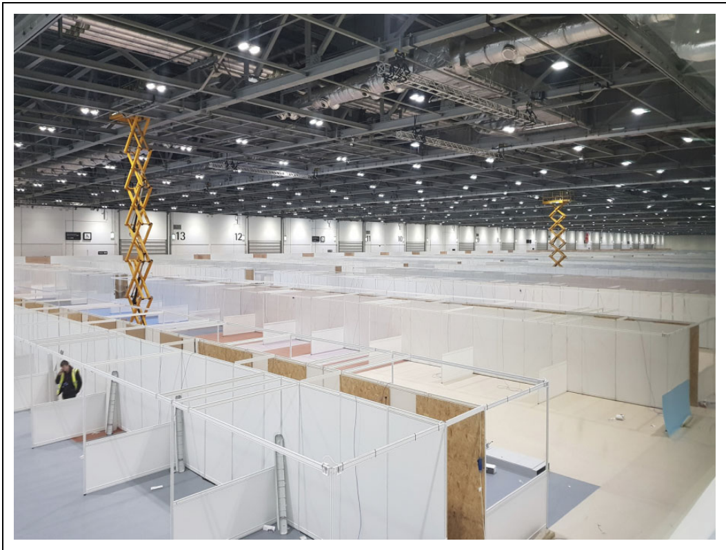
Figure 3. London ExCel Nightingale Hospital—Construction stage. Source: Images used with kind permission from BDP.
