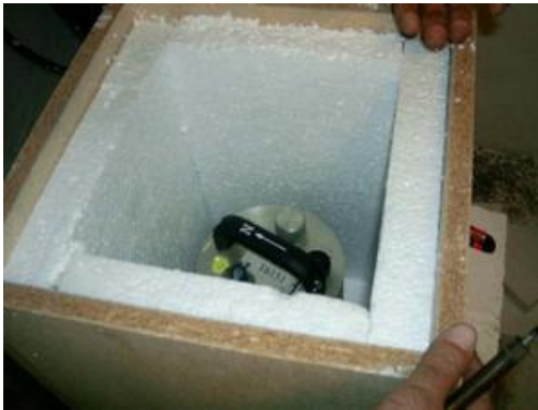
Figure 3.11: Broadband seismometer thermal insulation (inside installation)
