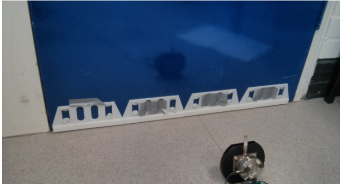
Figure 10 Base of Door with Devices fitted along the base of the door. The artificial ear is aimed at the gap through which sound flows.
