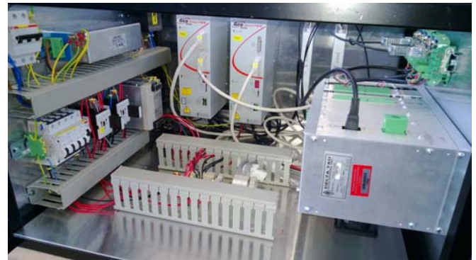
Figure 6. A picture of the electrical cabinet with the Power UMAC modular system.
