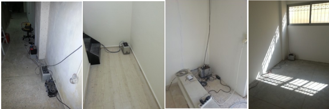
Figure K.1. Wired accelerometers
