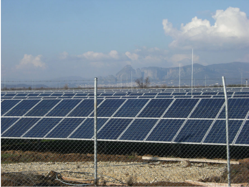
Figure 1. A photovoltaic park stands on the agricultural plain in western Thessaly, April 2014. The view is towards the UNESCO World Heritage Site of Meteora. (Photo: Daniel M. Knight.)
