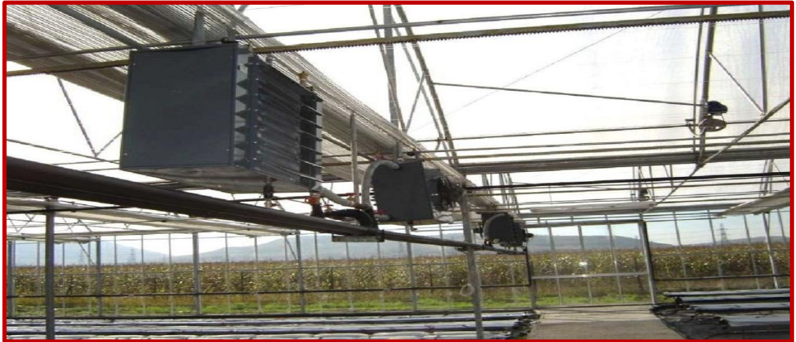
Figure 3:3 Hot water-charged air heater (Katsoulas & Kittas, 2009)
