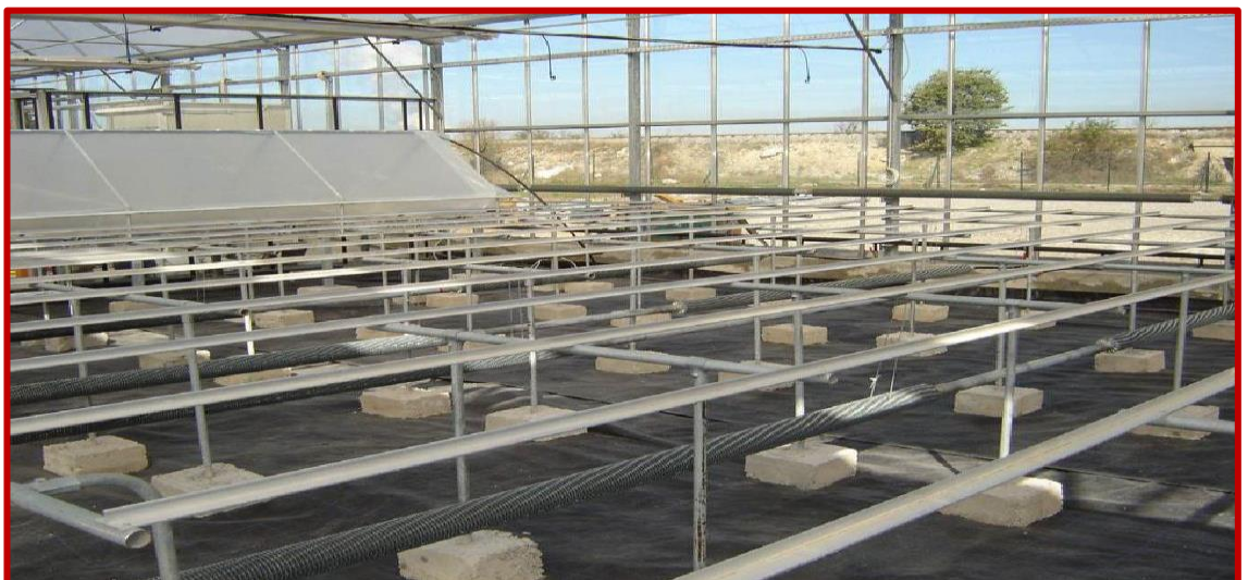
Figure 3:4 Hot water heating system with pipes installed under the plants beds (Katsoulas & Kittas, 2009)
