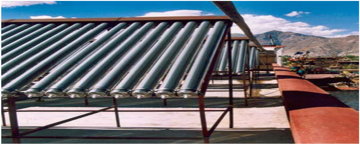
Figure 3:18 [11] Solar water heating system
