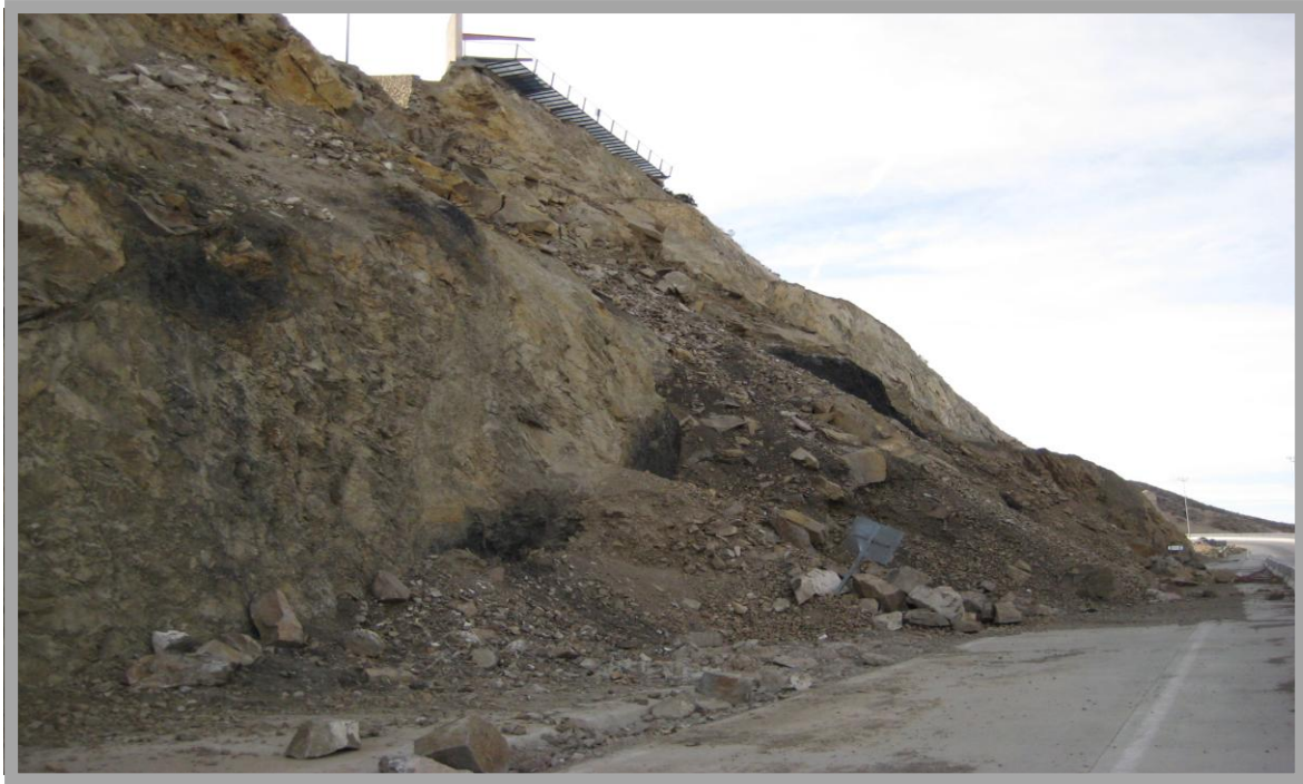
Figure 1.7. Landslide in July 2008 in the Camino Real road over a mountainous area of the road at position km 11+700. Note that the recent construction of this highway has led to instability of the surrounding rock mass, directly causing the collapse. The bedrock in this area is composed of metasediments in a nape sequence, and is heavily fractured, assisting collapse. Because of the weakness of the bedrock in the mountains, much debris was delivered into the city by flooding.
