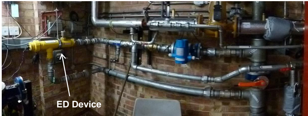
Figure 4.12: photograph of the device installation in the Halsbury Building, Brunel University.
