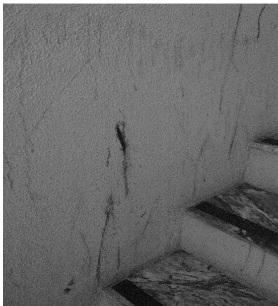
Fig. 7: Stained walls of stairs inside a rehousing building.
