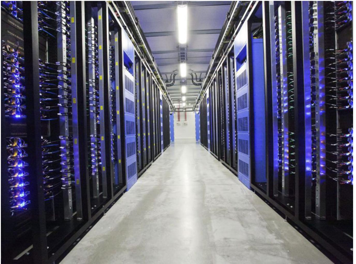
Figure 2.1: Core site data centre [3].
