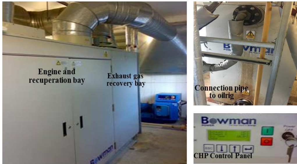
Figure 3.2 Combined heat and power unit
