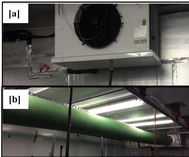
Fig. 2. Experimental test facility: [a] air distribution via plain evaporator coil and [b] air distribution via a round fabric duct.
