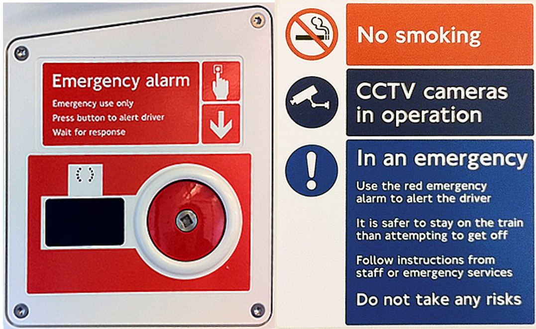
Figure 4.13 (Left) Emergency alarm in the Metropolitan line train
