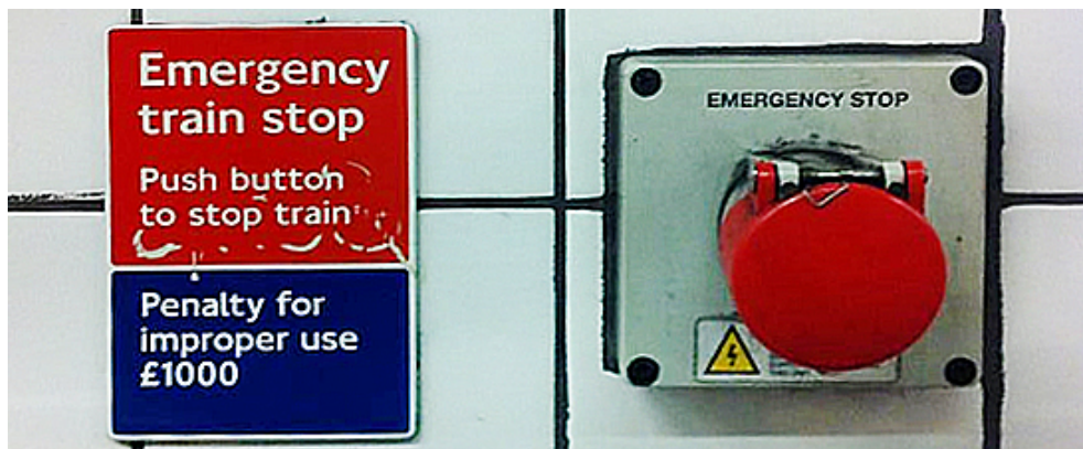
Figure 4.3 Emergency train stop button at platform at Oxford Circus station
