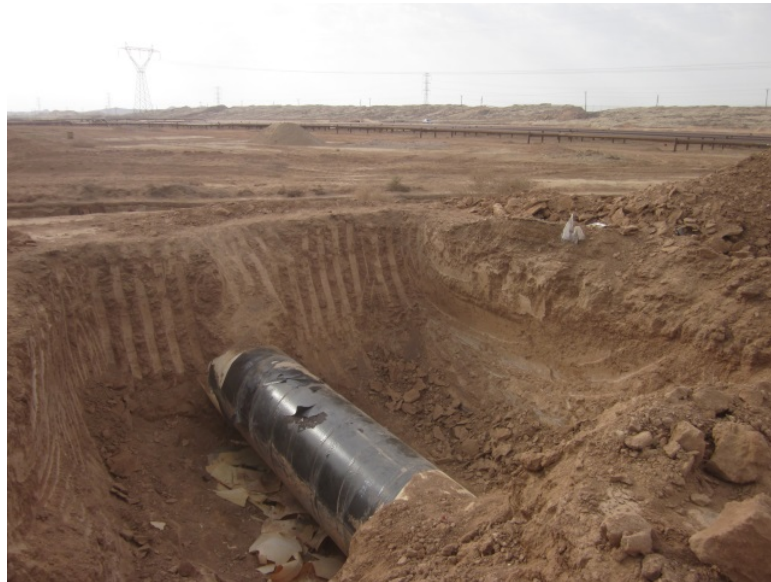
Figure 2-5: Examples of Direct Assessment. Picture on the top showed a coating defect detected at PR10. Picture on the bottom illustrates an example of an excavated site
