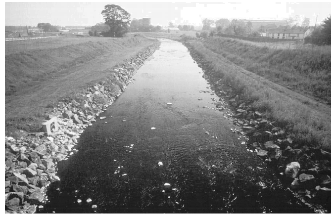
Figure 3. River Main: river channel and floodplains. Main channel is covered by cobbles, with medium rip-rap stones for the bank slopes and floodplains with natural grass.
