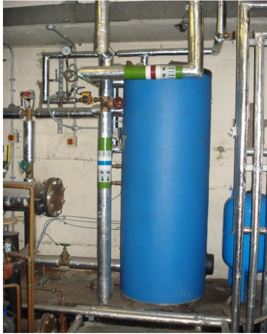
Figure 1.24 Calorifier fitted with appropriate thermal insulation. (Source: own collection)
