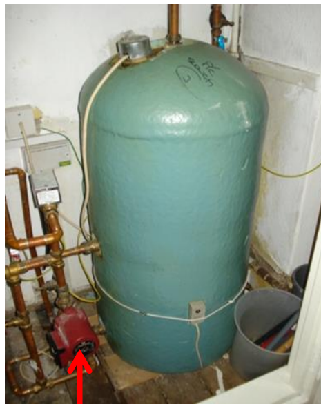
Figure 1.22 Calorifier fitted with circulating pump on the return pipework to maintain the temperature throughout the hot water system. (Source: own collection)
