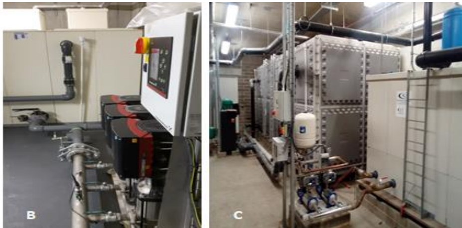
Figure 1.10. A – Schematic of a domestic hot and cold water system in W1T postcode (London) with mains break tank supplying the potable water; B and C are the typical examples of mains break tank located in the lower ground plant room connected to booster pump sets supplying potable water to the entire building. (Source: A-Own drawing; B and C own collection).
