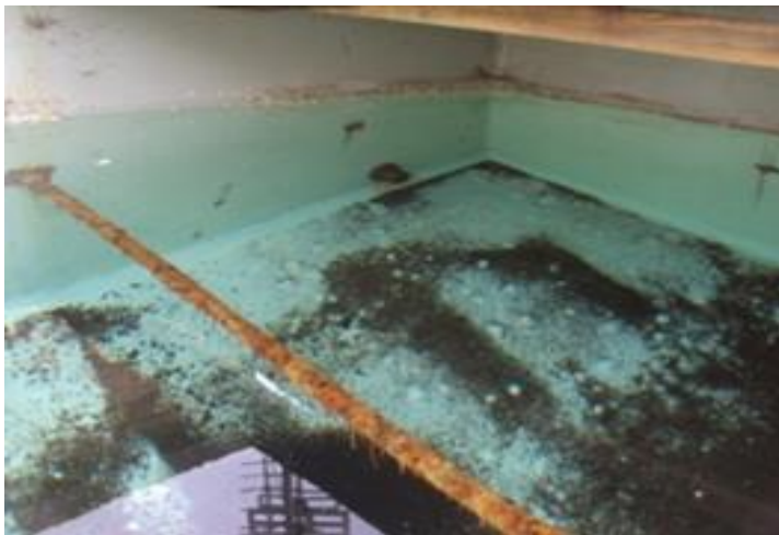
Figure 1.13 Sediments and corrosion at the bottom of a cold water storage tank (Source: own collection)
