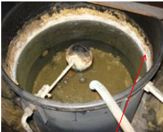
Figure 1.12 Scale accumulation on the tank wall (Source: own collection).
