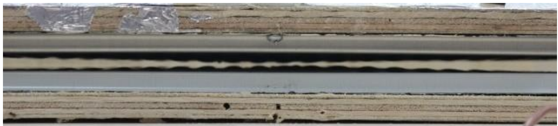
Figure 3.22 – panel expansion due to excessive heat supply
