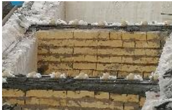
(c) Refractory pellet on the internal furnace wall
