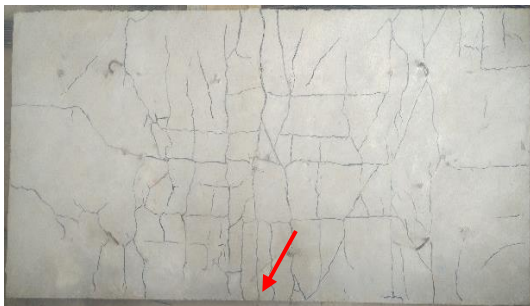
(c) Cracking pattern on the top surface
