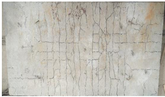
(a) Cracking pattern on the top surface
