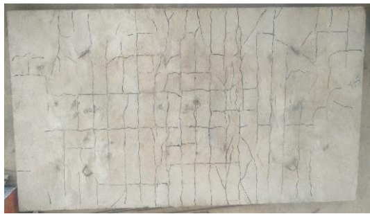
(a) Cracking pattern on the top surface
