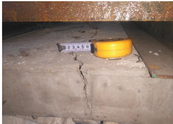
(b) Main crack
