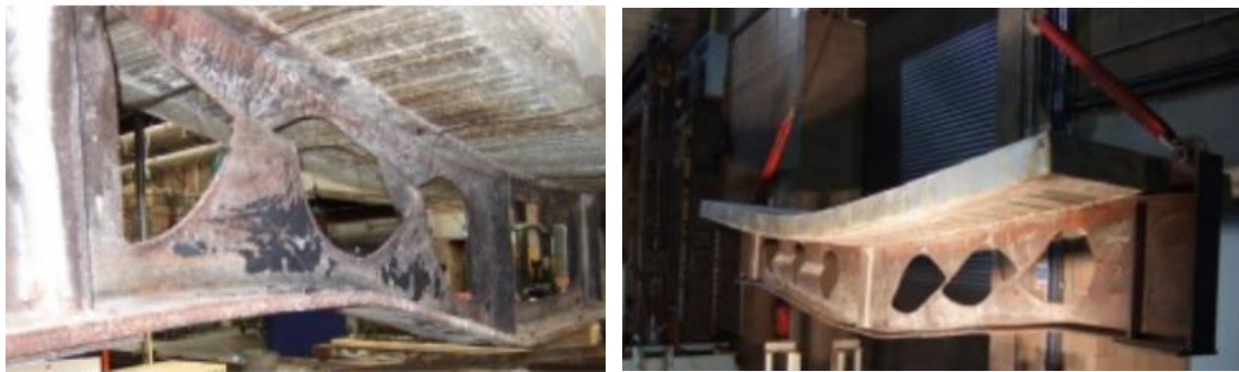
Fig. 2.13 Web-post buckling and Vierendeel bending in perforated beams exposed to fire (Nadjai et al. 2016)
