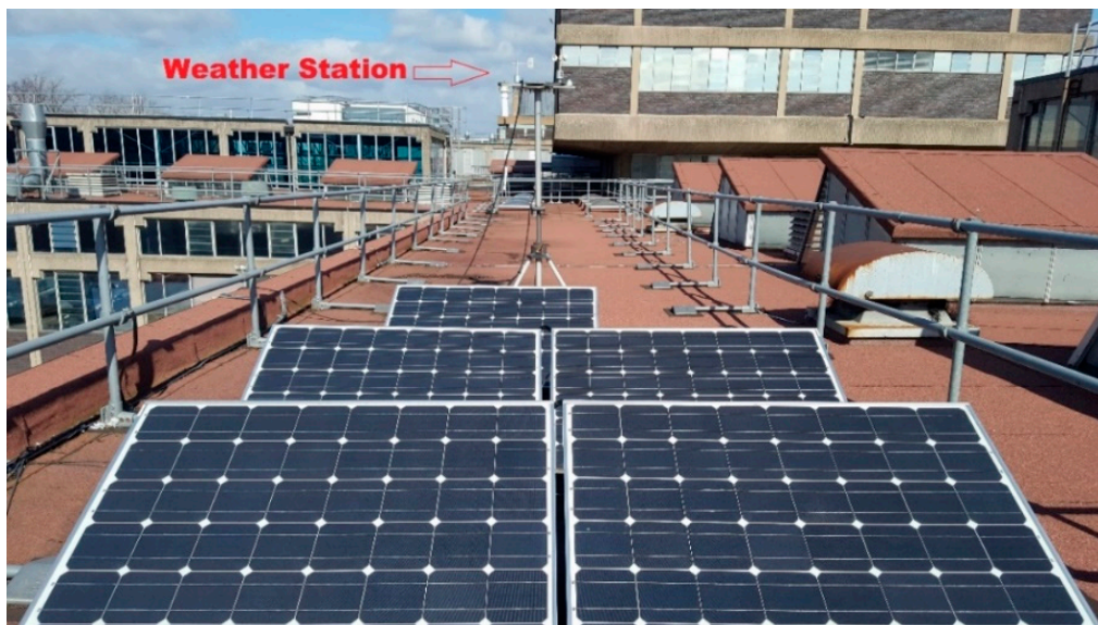
Figure 3. The studied PV array installed at Brunel University London, UK.
