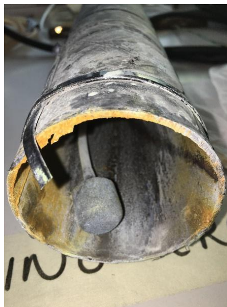
Figure 5.3: Example of pipe with Calcite and corrosion fouling attached to inner wall
