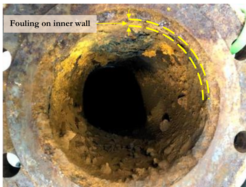
Figure 1.1: Example of fouling accumulation on inner wall of pipe specimen
