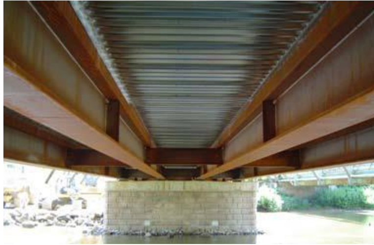
Fig. 1.8 Lynch Village Bridge (NSBA, 2012) as an example of composite bridges comprising concrete filled tubular flange girders (CFTFGs)
