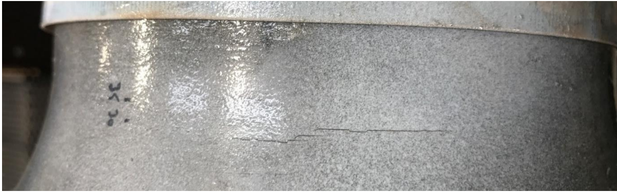
Figure 4-13 Crack Image taken with a mobile camera
