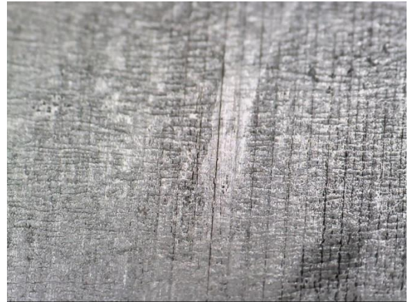
Figure 4-10 Crack image at 7th iteration from same area
