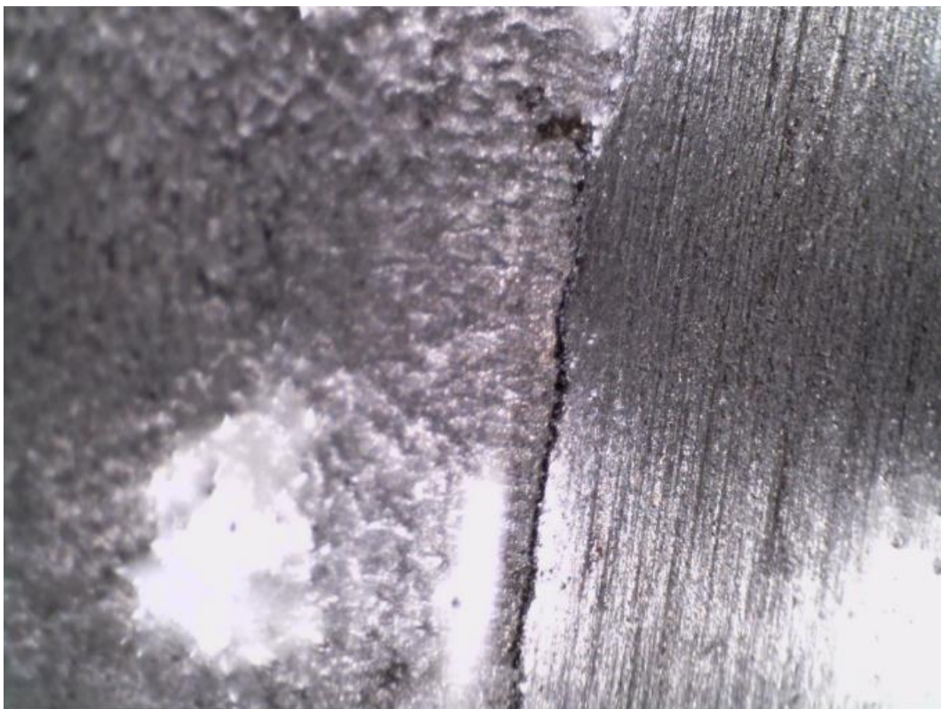
Figure 4-31 Site image indication at interface between corroded and finished areas
