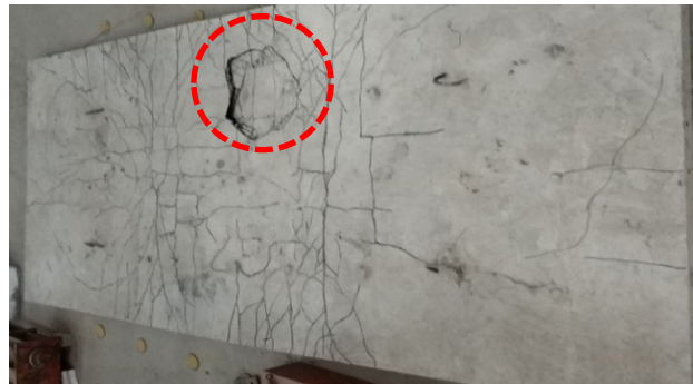
(a) Cracks on the top surface
