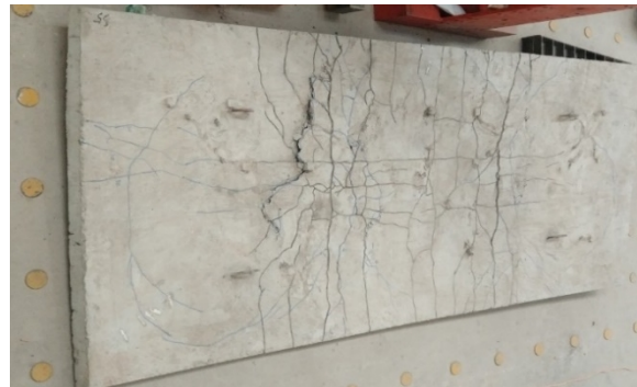
(a) Cracks on the top surface
