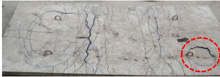
(a) Cracks on the top surface
