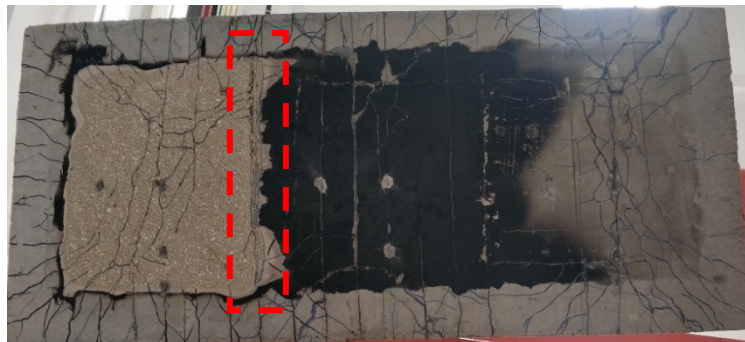
(c) Cracks on the bottom surface
