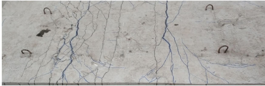
(a) Cracks on the top surface
