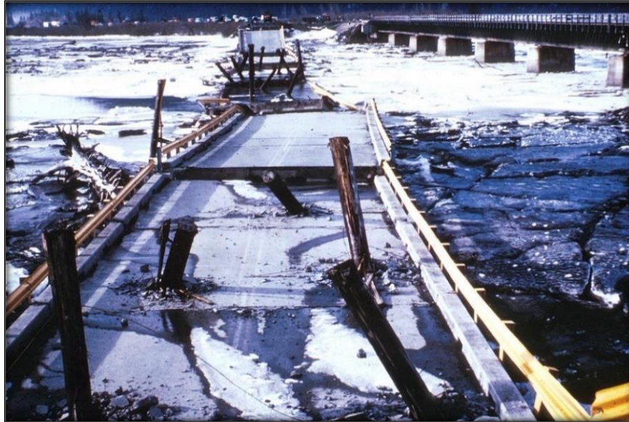
Figure 2-52 Concrete Deck of Bridge 629 that Collapsed due to Penetration by Timber Piles, (Dickenson, Barkau & Wavra, 2002)
