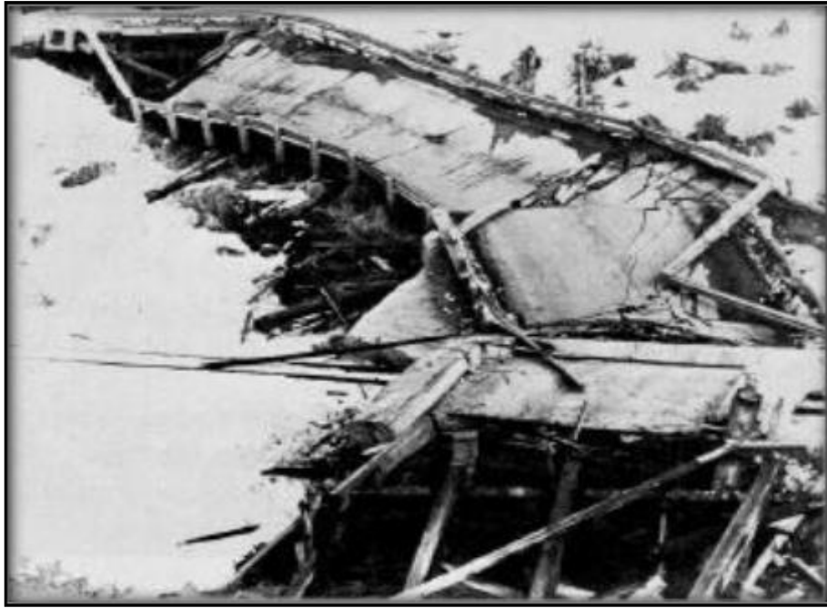
Figure 2-50 Snow River Bridge 605 Collapse due to Liquefaction, (Ross, Seed & Migliacio, 1973)
