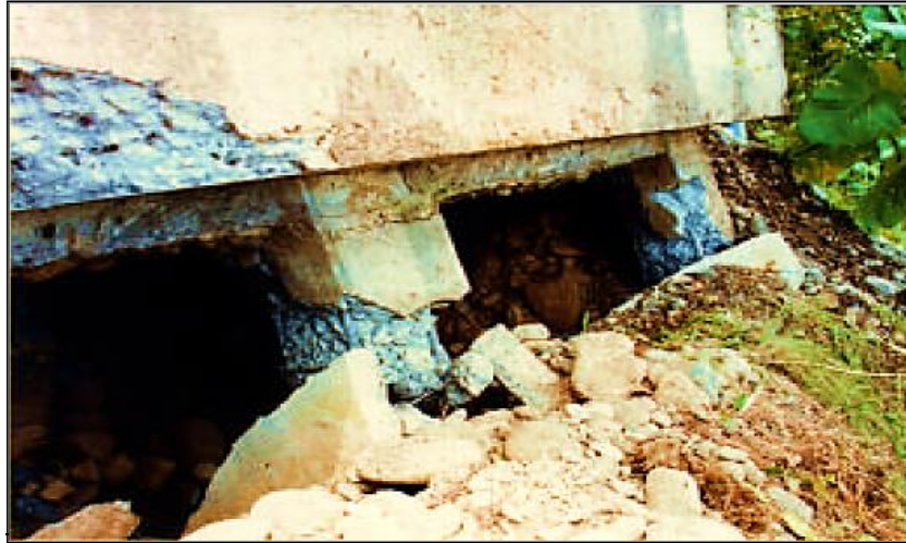
Figure 2-72 Differentiation Damage Induced to Front Batter Piles of Rio Banano Bridge, (Ravazi, Fakher & Mirghaderi, 2007)
