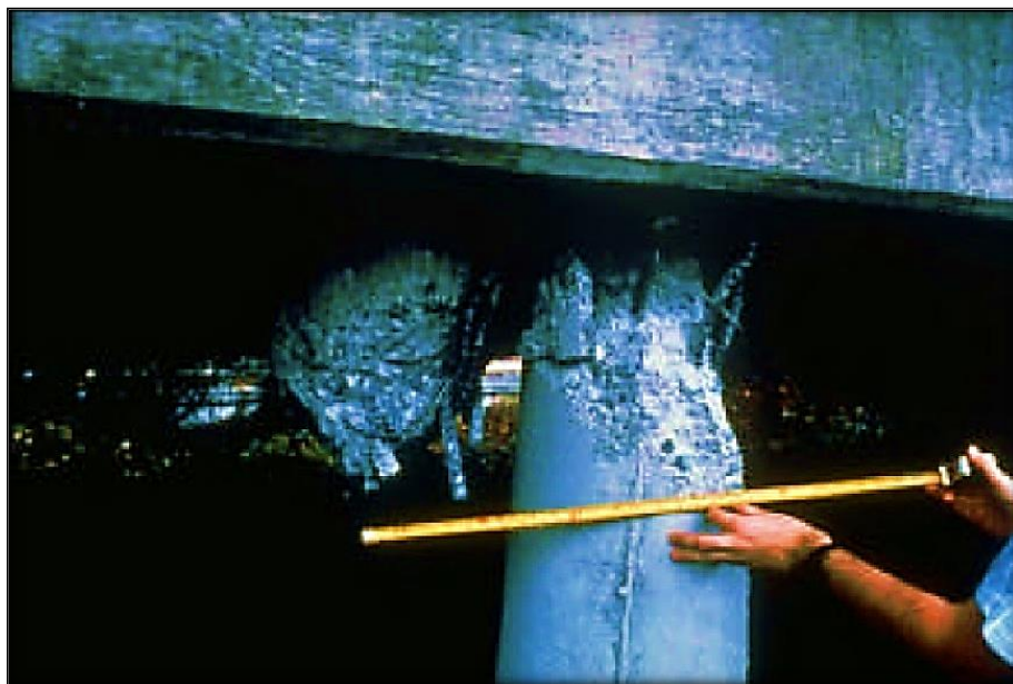
Figure 2-70 Flexural Shear Failure of Pile-Bent Connection of the Struve Slough Crossing, (Seed et al., 1990)
