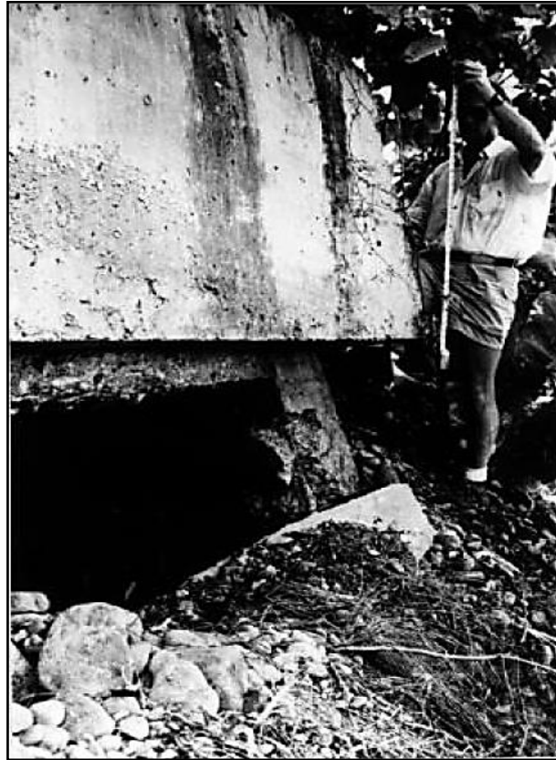
Figure 2-71 Rotation of Rio Banano Bridge Pile Cap, due to Liquefaction, (Ravazi, Fakher & Mirghaderi, 2007)
