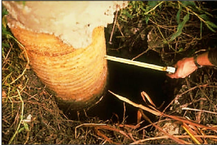
Figure 2-69 Creation of Gap Between the Soil and One of the Piles Supporting the Collapsed Struve Slough Crossing, (Seed et al., 1990)
