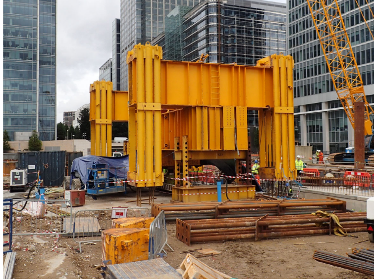
Fig. 2 Static load testing frame for the trial test pile (reproduced from de Battista et al. [29] with permission).
