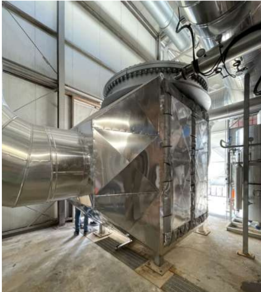
Figure 18: Photograph of a pressurised HPHE for recovering energy from a ceramic roller kiln.
