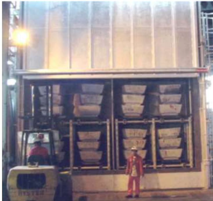
Figure 5: Photograph of an aluminium sow preheater using exhaust gases [24].
