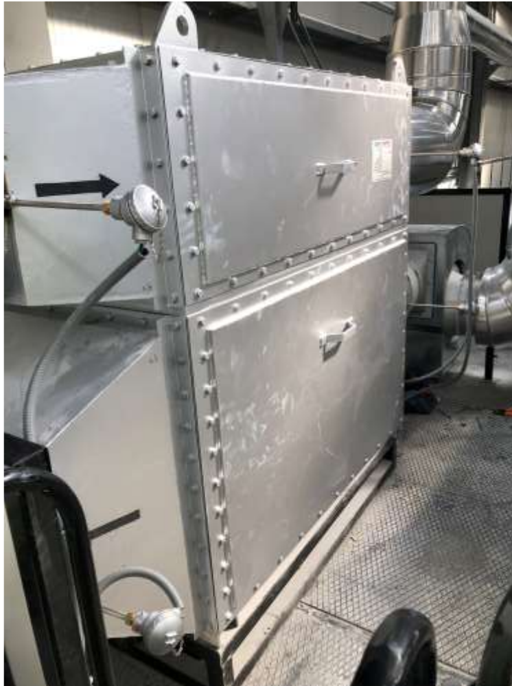
Figure 55: Experiment 2 installed HPHE photograph.
