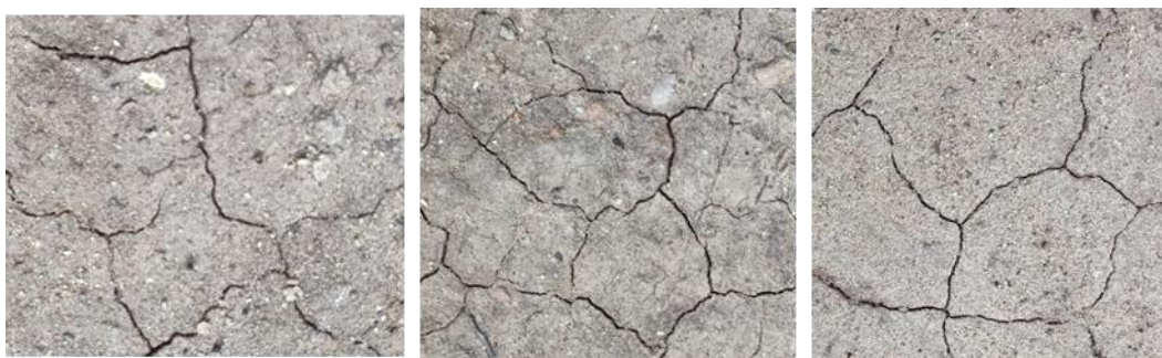
Fig. 5: Sample Images of Soil Shrinkage Cracks
