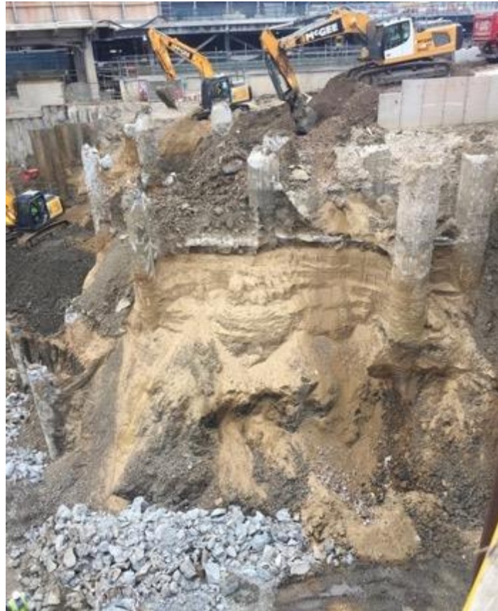
Figure 4. 1 – An excavation at Battersea Power Station with the previous structures piles exposed. Showing additional implications for site investigations and developing a site that has been previously developed.
