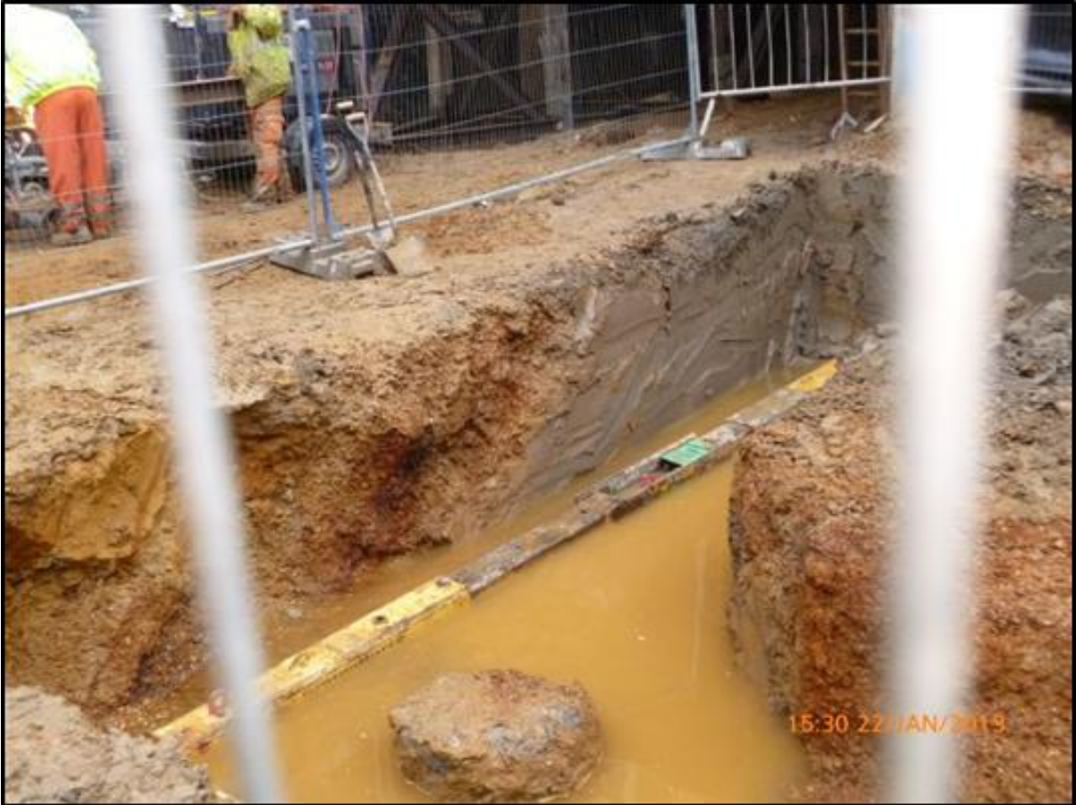
Figure 9.8 – Inclined contact between DFH infill to the left and London Clay to the right.
