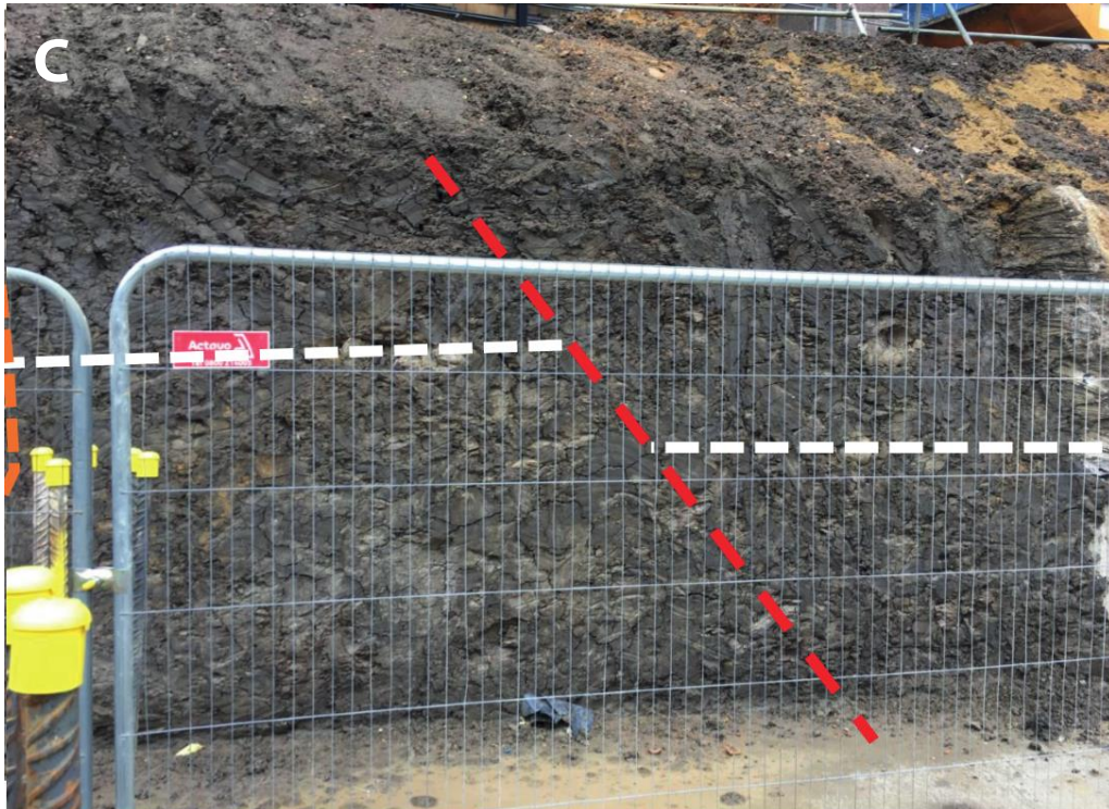
Figure 9.6 – Offset London Clay at the edge of the Battersea Phase 3a feature.
