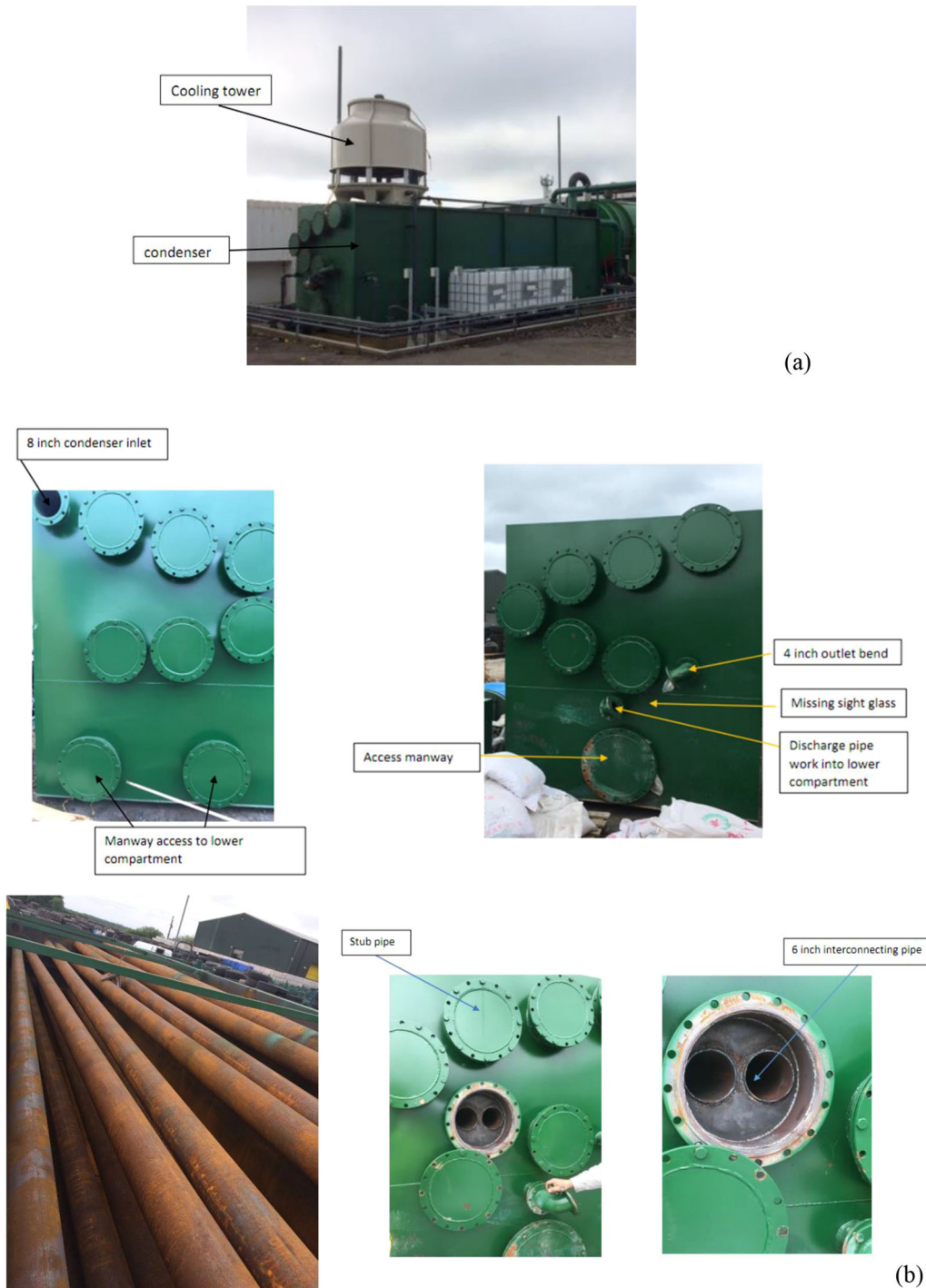
EXHIBIT 2 The photo of (a) the condenser with a cooling tower and (b) components of the condenser with details. [Color figure can be viewed at wileyonlinelibrary.com ]
