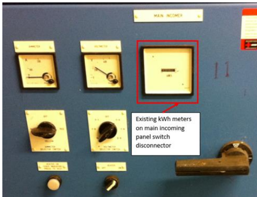
Figure 3-3 Existing Analogue Power Meter
