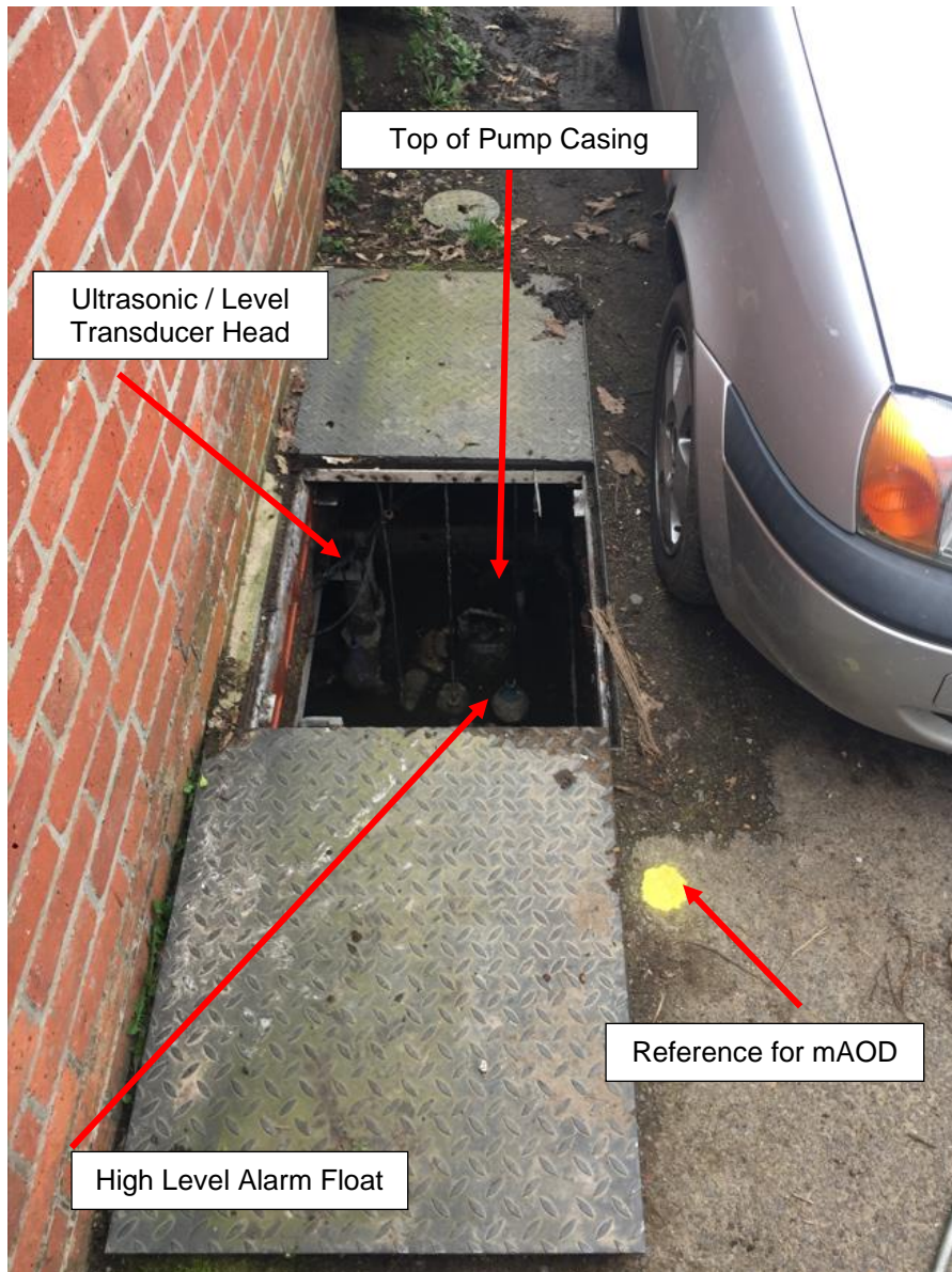
Figure 5-6 Example wet well from photo taken during surveys
