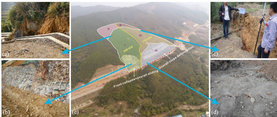
Fig. 2 On-site investigation of the landslide area: a landslide bed, b shear outlet, c steep scarp and d uplift of road surface
