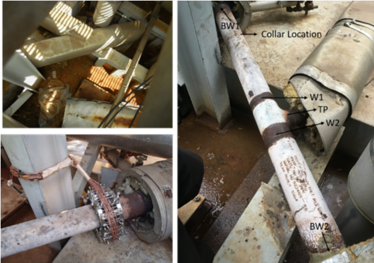
FIGURE 6.17: Installation of the transducer array in an operational power plant showing the installed location and key pipe features.
