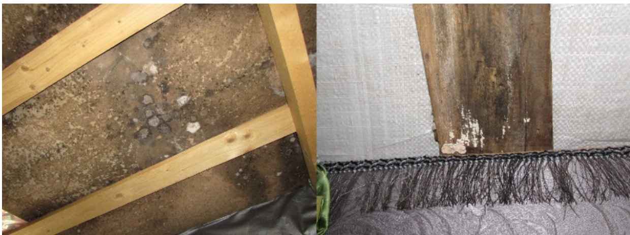
Figure 3. Example of mold growth on the ceiling ( left ) and wall ( right ) wood panels inside informal settlements.
