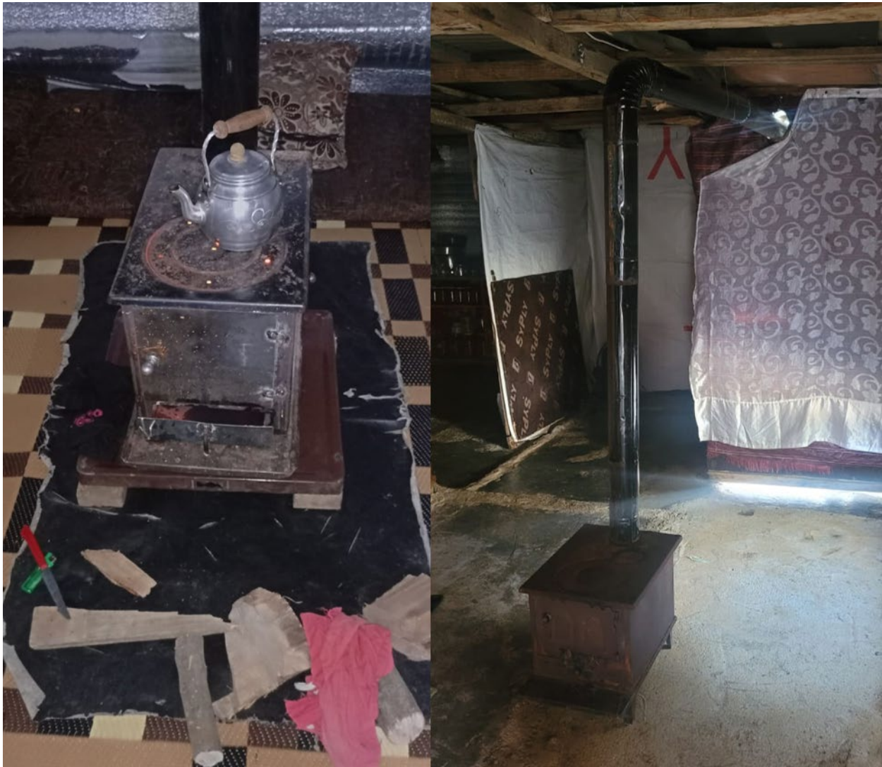
Figure 6-1. Heating in ITS. Kerosene stove serving a living area inside informal tented settlements in the Bar Elias Syrian Refugee camp.
