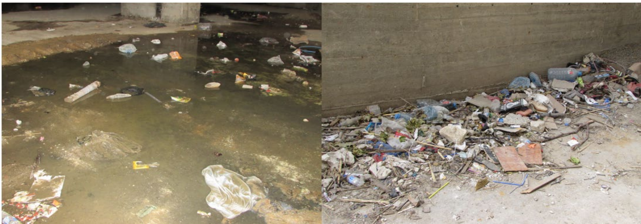
Figure 3-6. OUC Hygiene Observations. Sewers leaking in OUC basement (left). Unmanaged waste outside the OUC (right).
