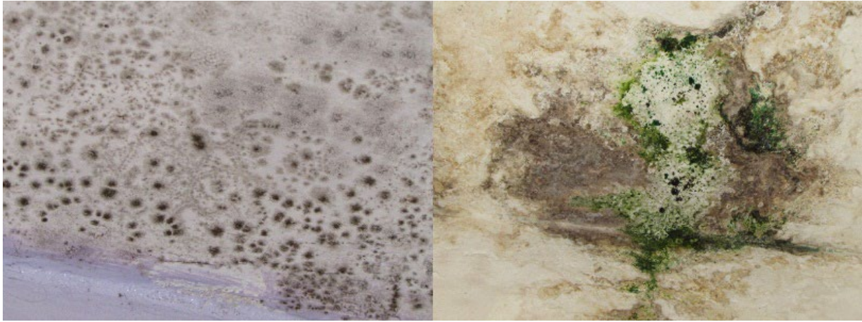
Figure 4-3. Mould in Residential Shelters. Examples of evident sporadic (left) and concentrated (right) mould growth on residential shelters ceilings.
