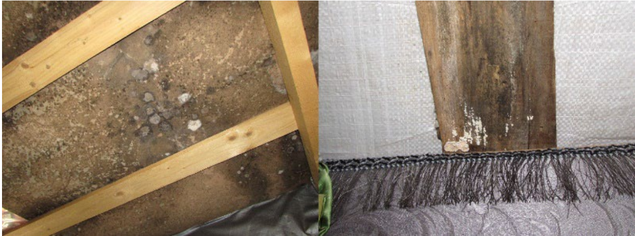
Figure 4-4. Mould in Non-permanent Shelters. Example of mould growth on ceiling (left) and wall (right) wood panels inside informal settlements.
