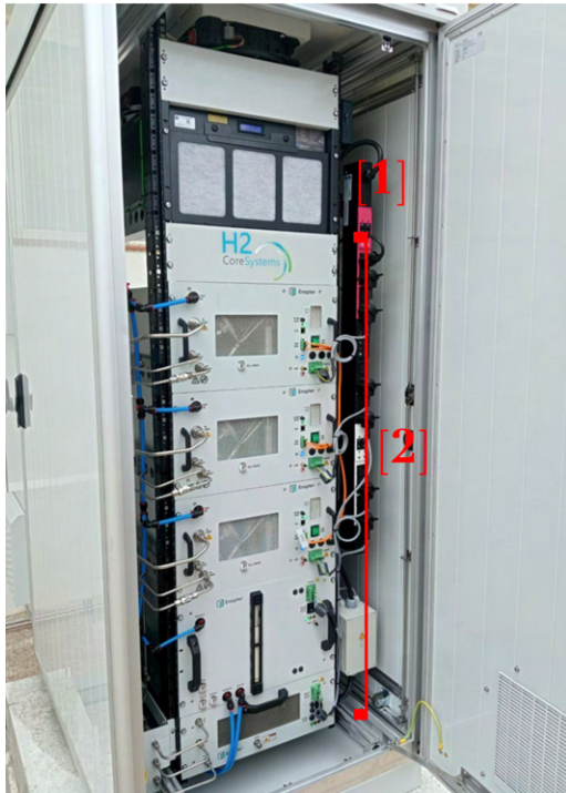
(a) The hydrogen system cabinet consisting of the [1] the 4kW fuel cell and [2] the 7.2kW electrolyser stack.
