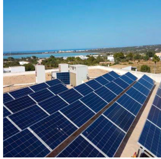
(b) Current solar capacity installed on the roof of the small school
