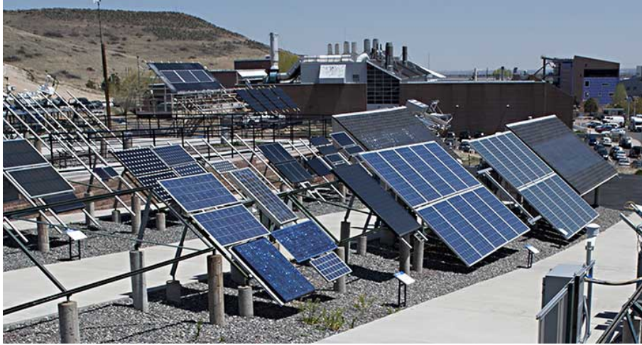
Figure 4.1: NREL PV solar test set up in Golden, Colorado.
