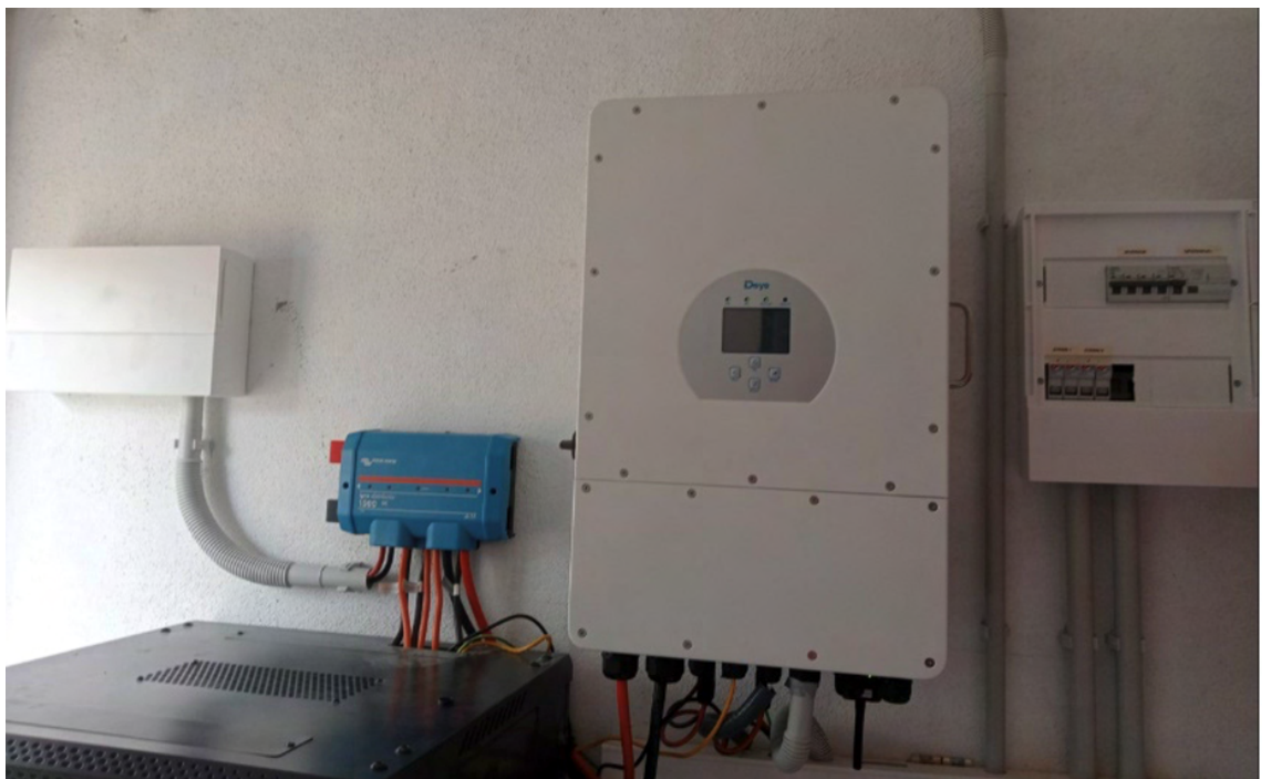
Figure A.4: The 15kVA three-phase inverter and 48V DC bus to manage the DC power generation and battery storage for the REC system.
