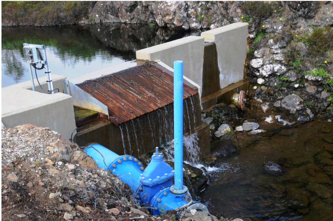
Figure 2.14: small-scale hydroelectric generator located on the Isle of Eigg [63]
