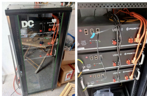
(b) Battery cabinet housing the 14.4kWh stack
