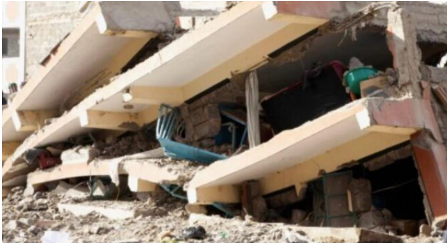
Figure 1.2 Building collapse in Akyem-Batabi (Frimpong, 2020)
