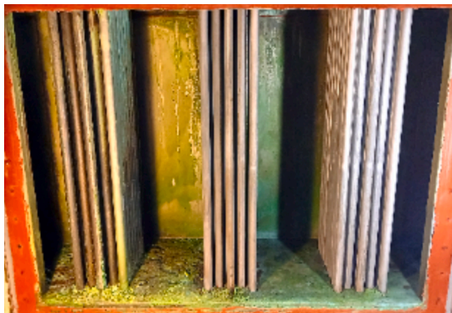
Fig. 19. Internal surfaces of the condensation unit after experiments.
