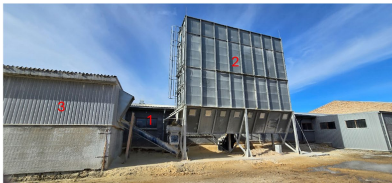
Fig. 2. Sanding dust extraction system; (1) panel treatment facility with cutting and sanding equipment; (2) Dust filters and separators; (3) sanding dust storage room 43,44 .
