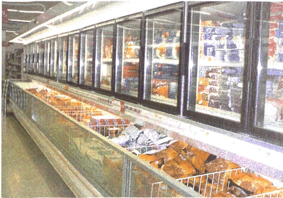
Figure 2.3 - Horizontal Well Type Case with Glass Door Reach-ins Above
