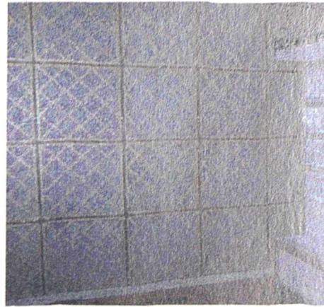
Figure 3.6 - Return Air Plenum Wall
