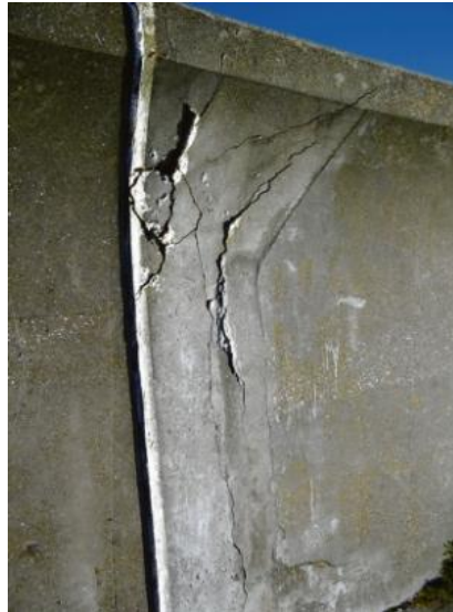
Figure 1.2: Canvey's seawall in Essex, England is cracked due to high pressure arising from wave breaking on the wall. (image taken from http://www.echo-news.co.uk/ )
