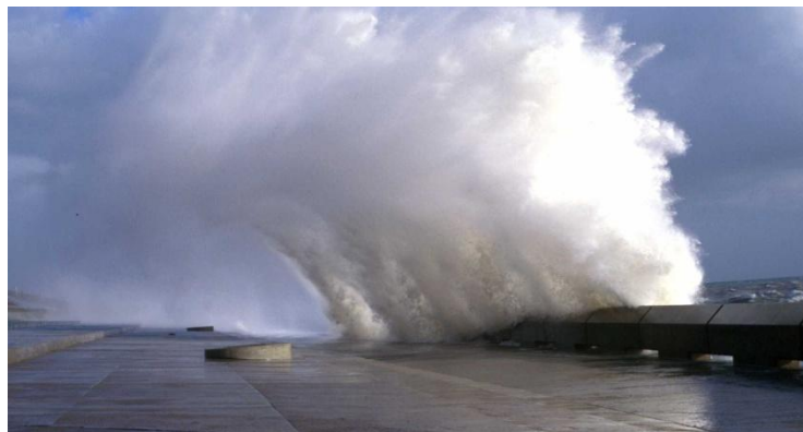
Figure 1.4 : Violent wave overtopping at the Samphire Hoe seawall, UK, taken from CLASH project, http://www.clash-eu.org .
