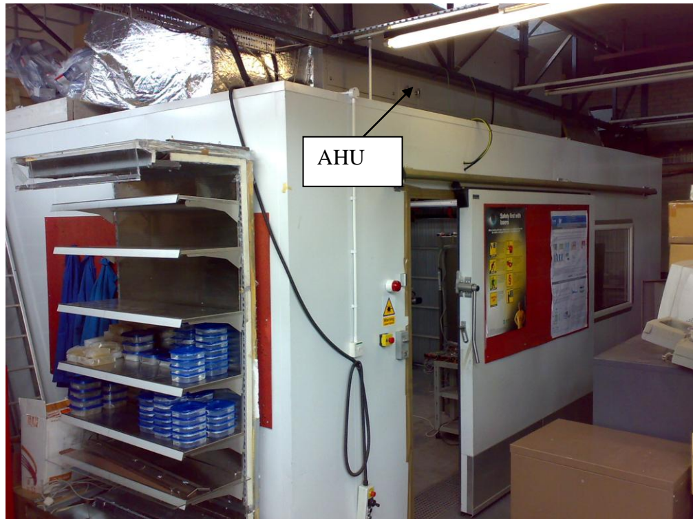
Figure 3.4 General arrangement of the test room and the air handling unit
