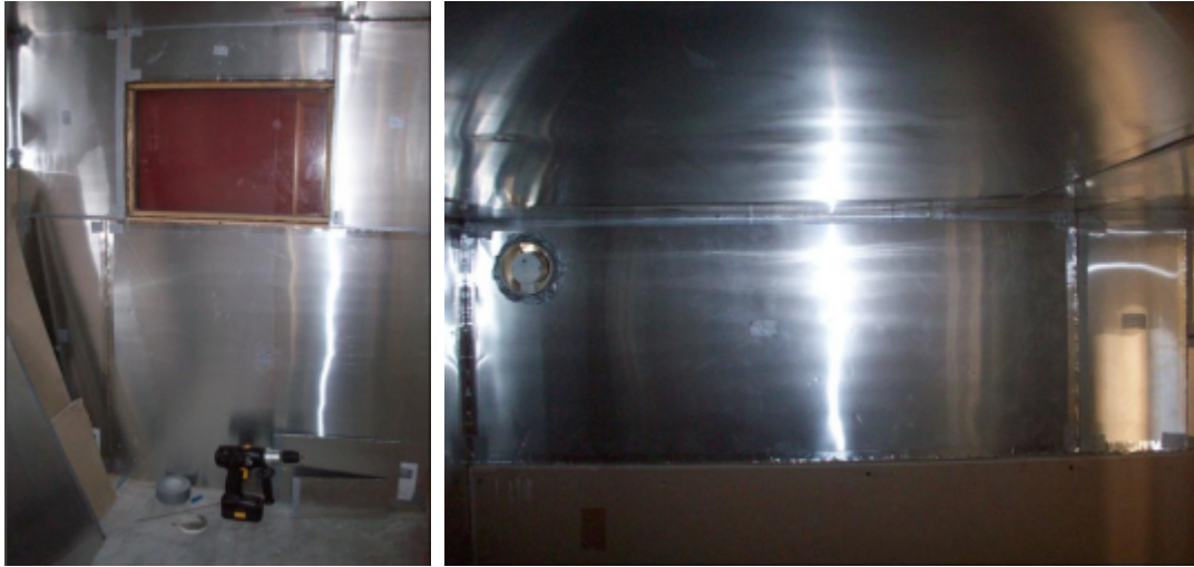
Figure ES.16 Energain panels applied to the internal surfaces of the test cell.
