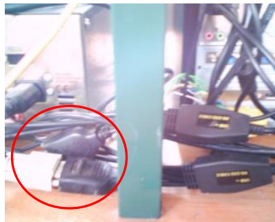
Figure 8-22 USB-to-RS232 converter cables connected to RFID readers
