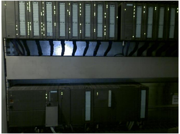
Figure 9-14 PLC in charge of side-panel manufacturing central control
