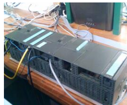
Figure 8-15 Siemens S7-300 PLC device
