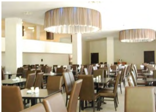
Figure 13 Lighting installation in the restaurant area
