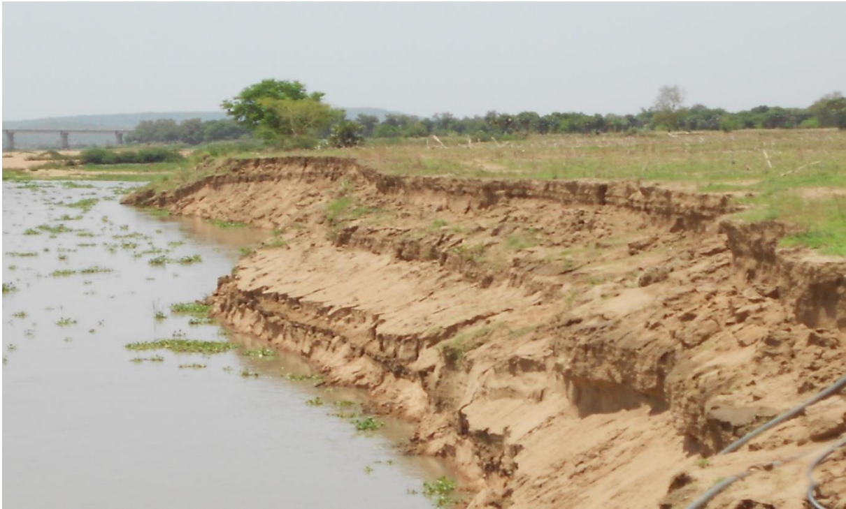
Figure 2.9: Land loss as a result of persistent erosion and collapsing of River Benue bank, due to river flow and seasonal flooding at sampling location E, see Figure 2.8 (The photograph taken by the author on 24 th April 2012).
