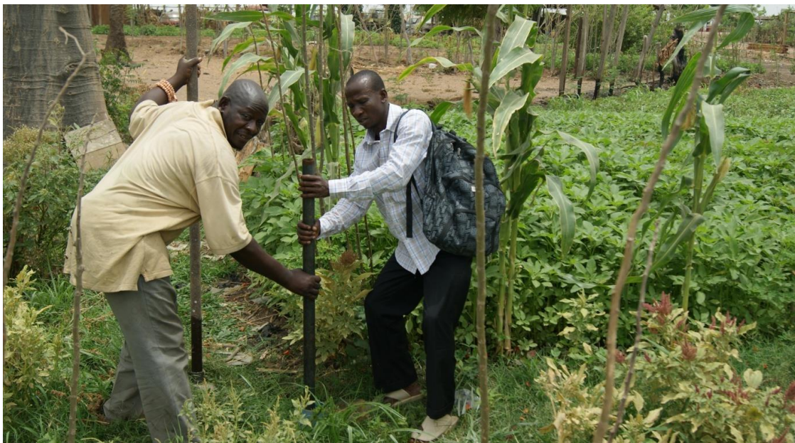
Figure 2.22: Pulling pipe out of borehole drilled with locally hand drilling augering method in the study area (The photograph taken by Mohammed Abana Girei on 15 th April 2011).
